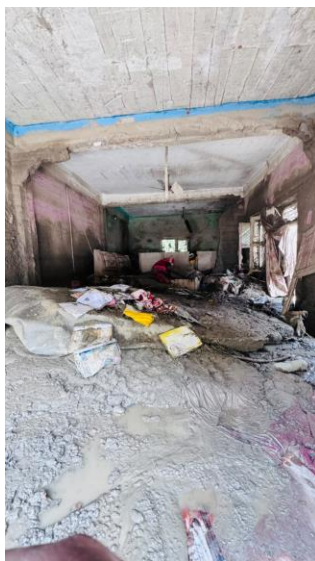
Bipin Malla's residence filled with flood debris.
